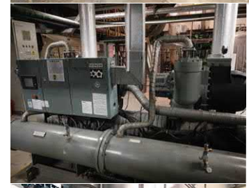
A/C Water Recycle System
