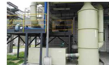
Spray tower for odor removing
