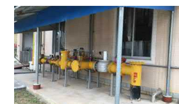
Natural gas pipeline
