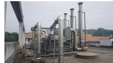
Biological VOC treatment Devices
