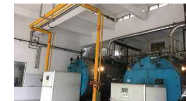
Natural gas remodelled boiler
